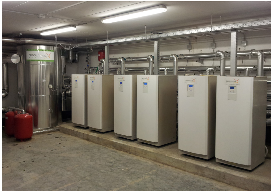
The heating room with Thermia Robust ground source heat pumps
